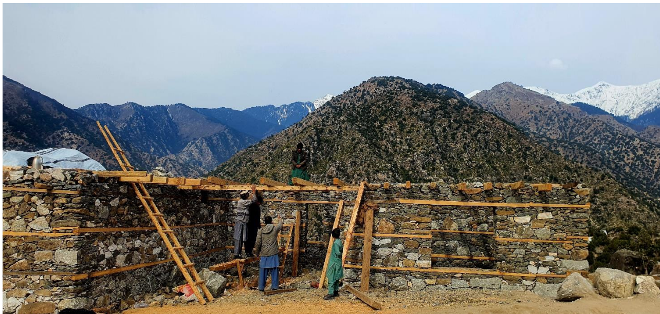
Photo 5. Community members work to re-construct their homes through the cash and technical support provided by DRC.
